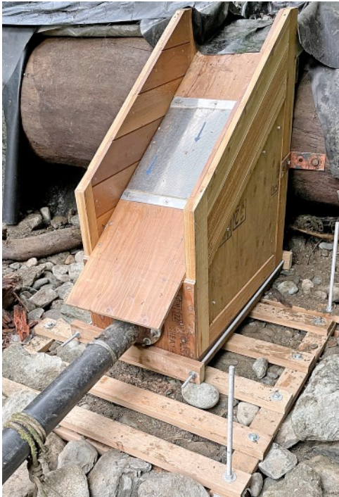
Marble Creek Intake Box
